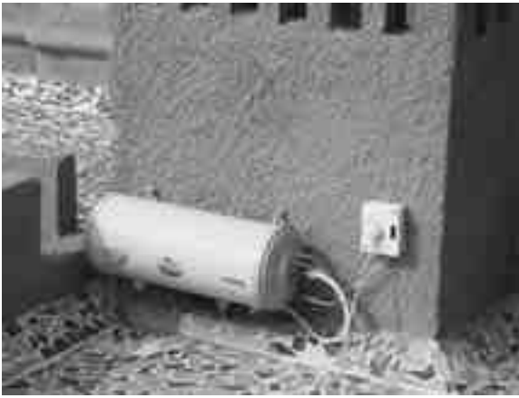
Fig 51: Electric geysers at Maple, big electricity consumers
